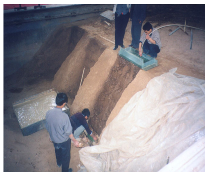
(a) 坡面汇水冲刷
